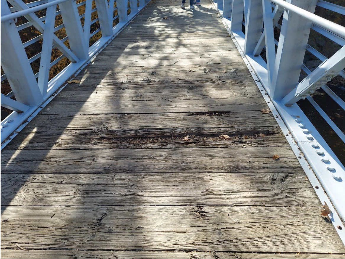
Pedestrian bridge surface damage, north end
