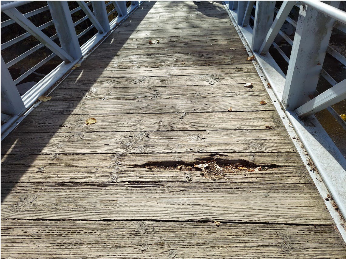
Pedestrian bridge surface damage, south end
